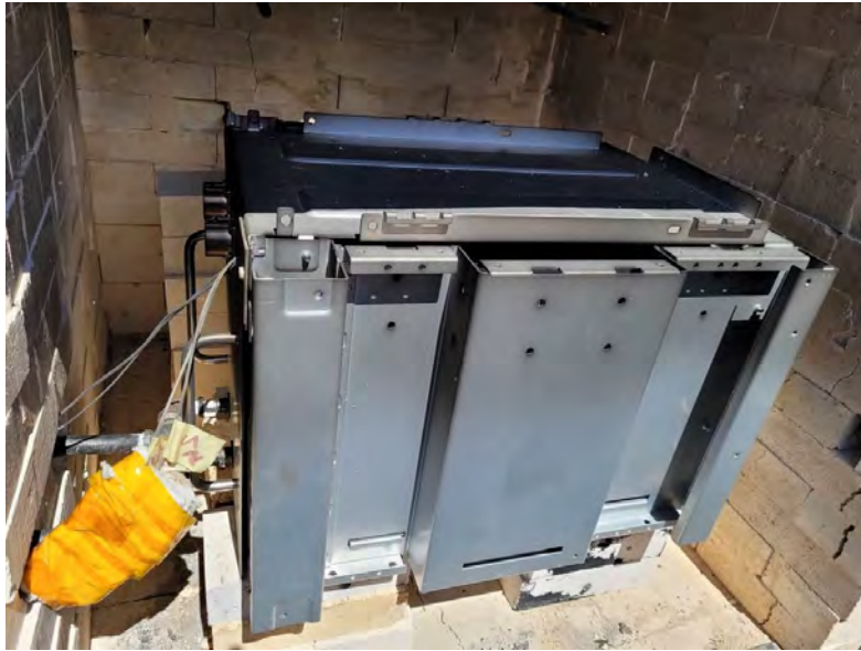
Picture 7 – Unit BBU – Unit After Exposure at 215°C
