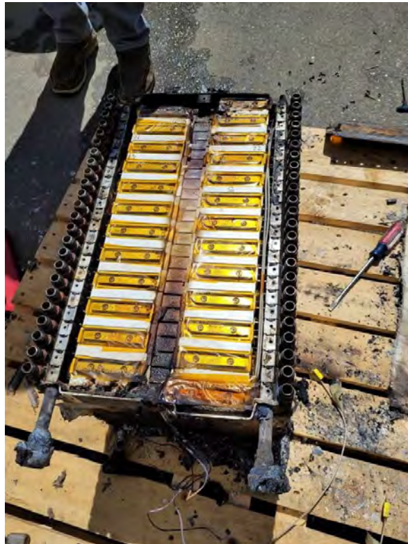
Picture 16 – Unit BBU – Unit After Exposure at 950°C – Top Protection Panel Removed – Exposed Battery Top Cells
