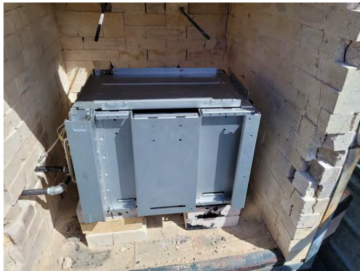
Picture 6 – Unit BBU – Unit Installed in the Test Chamber
